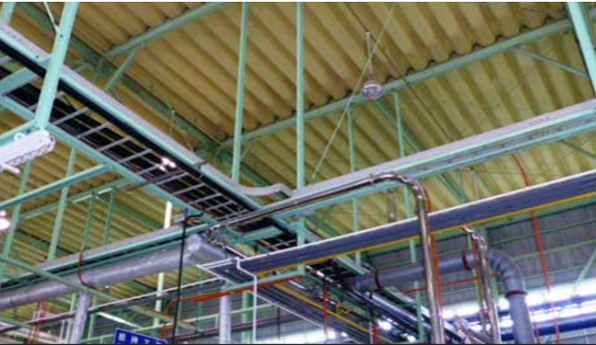
Falling object countermeasure, wiring rack anti-sway
