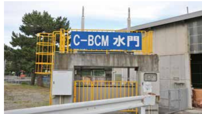
Sluice gates for tsunami countermeasures
